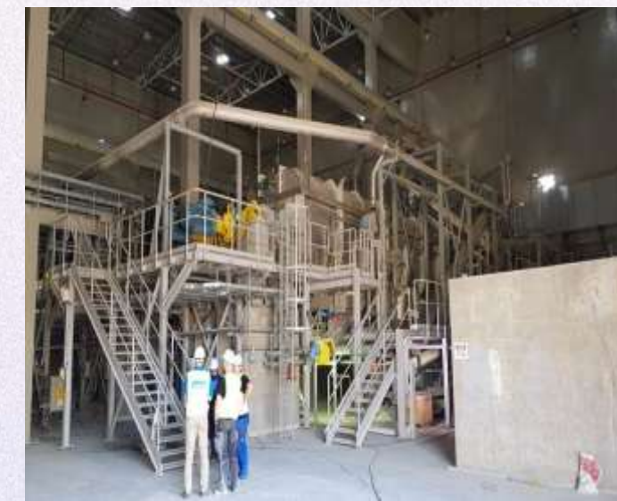
Jebel Ali Sewage Treatment Plant
