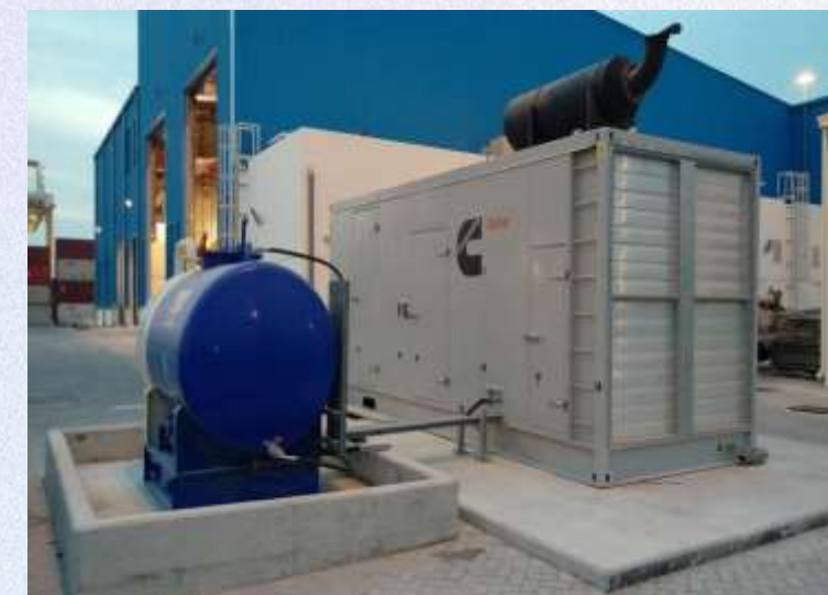
500KVA Acoustic Enclosure and Fuel Storage Tank
