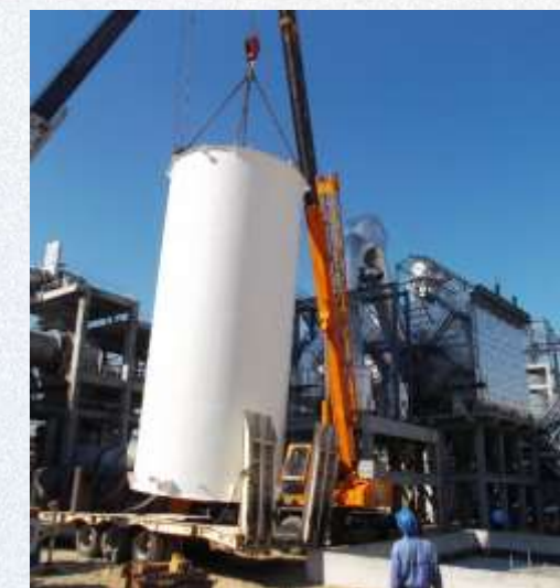
91,000 LTR Fuel Systems – Ammonium Hydroxide Tank
