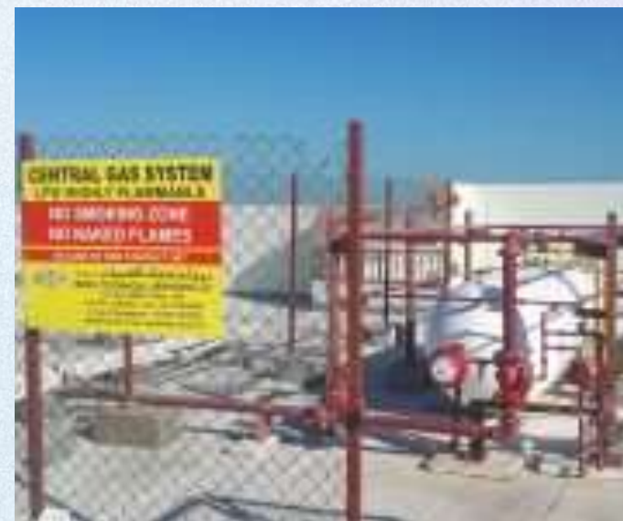
LPG Tank and Piping
