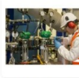
Operation and Maintenance Services
